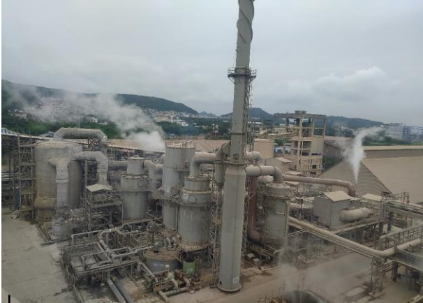
1400 MTPD Sulfuric Acid Plant I
