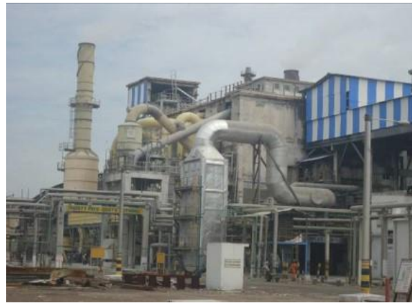
2100 MTPD Complex Plant Train A & B
