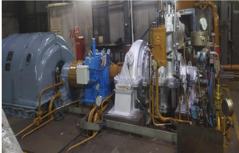
Turbo Generator - I 5 MW Condensing Turbine
