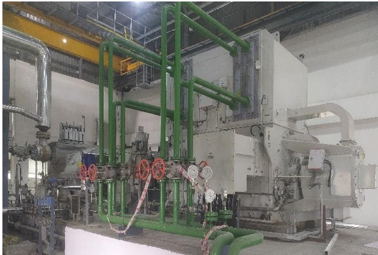
Turbo Generator - III
