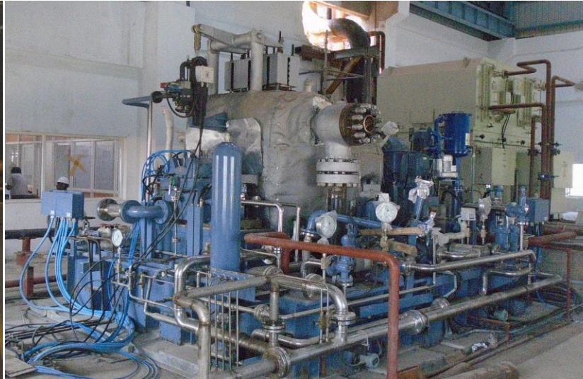
Turbo Generator - II 6.5 MW Non-Condensing Turbine
