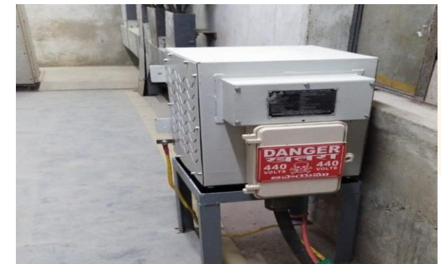
Central & Field Capacitor Banks
