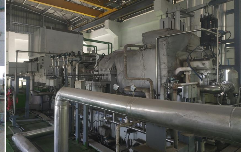
Turbo Generator III 15.25 MW Condensing Turbine
