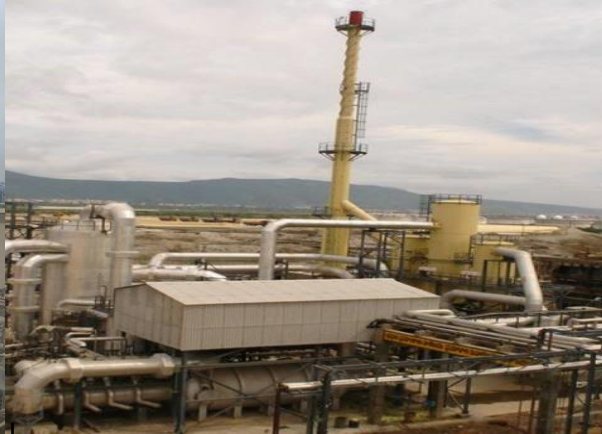
400 MTPD Sulphuric Acid Plant II
